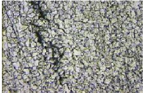
Fig. 7 Microstructure shows cracking (X200)
